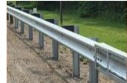
Metal Beam Crash Barrier
