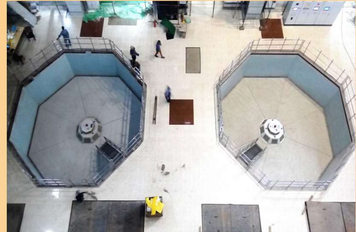
Power House, Umtru
