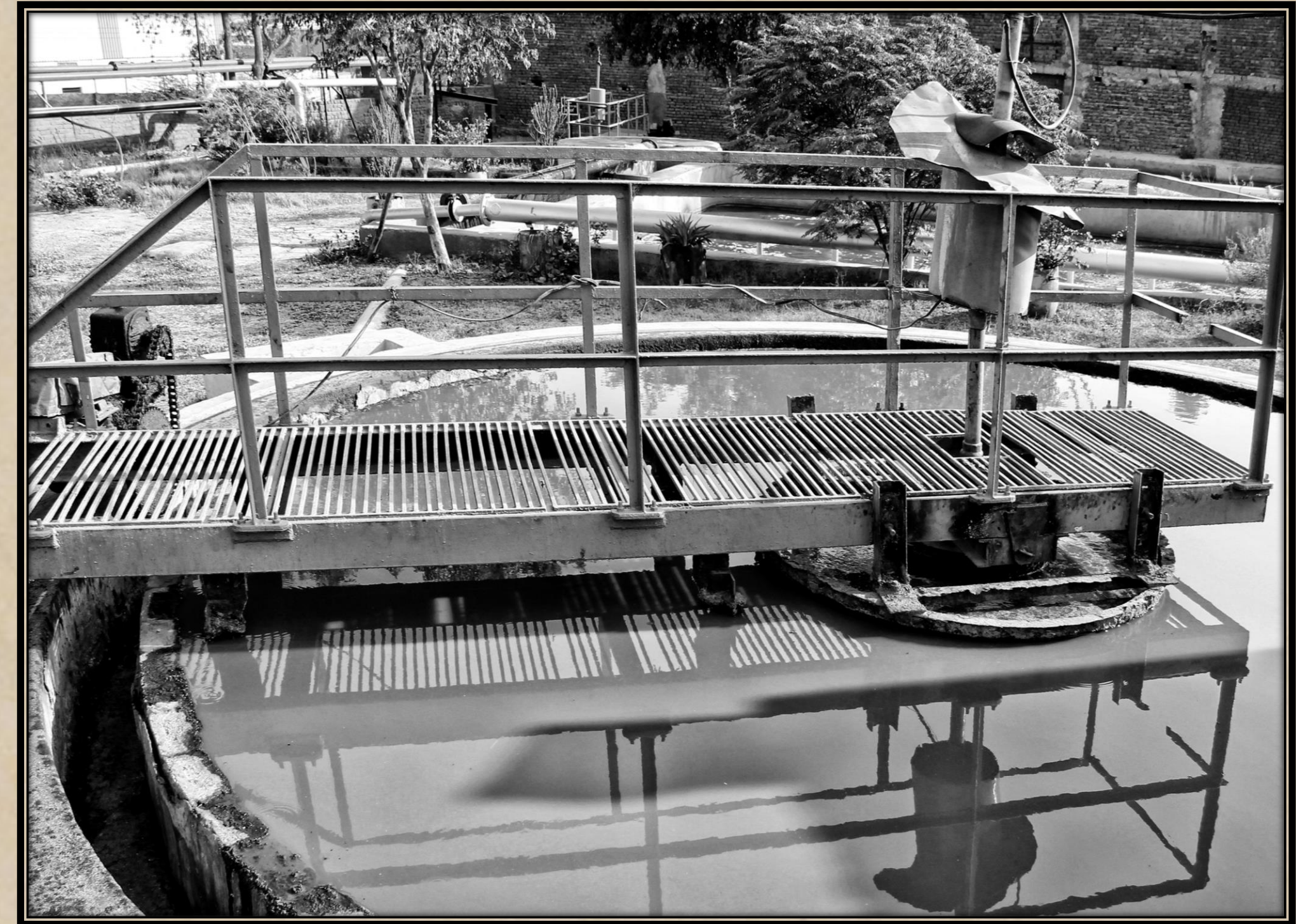
Effluent Treatment Plant - Our ETP is based on Activated Sludge process, adopted internationally all over world in Pulp & Paper Industry. It consists of Equalisation tank, Saveall, Primary Clarifier, Aeration and Secondary Clarifier.
