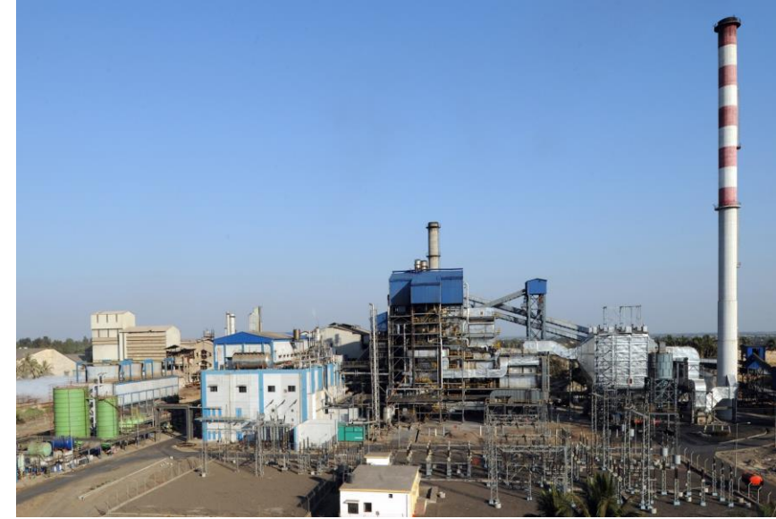
36 MW Power Plant on EPC basis at Shirol, India
