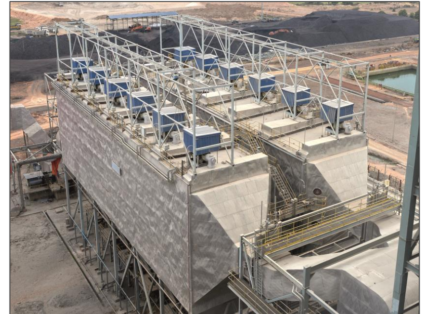
ESP, Power Plant for Bhubaneswar Power Pvt. Ltd., India
