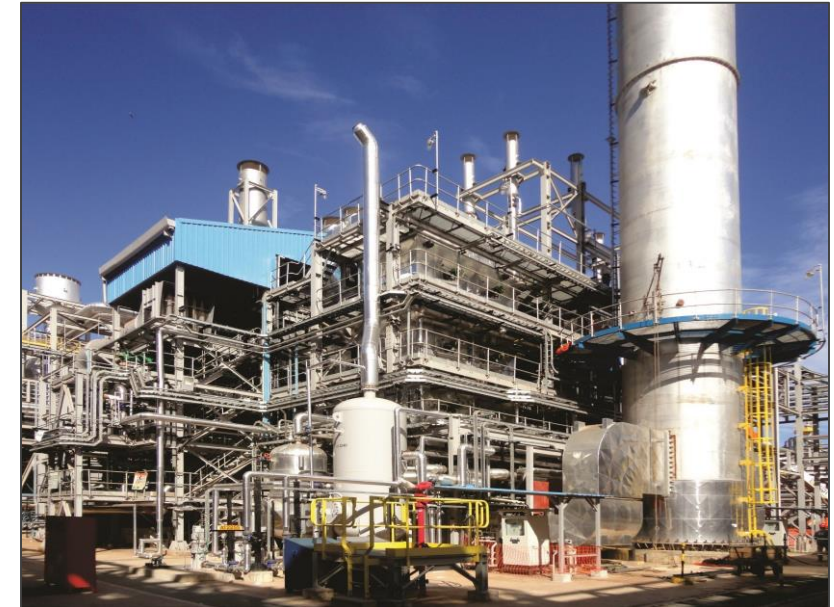
Oil & Gas Fired Boiler
