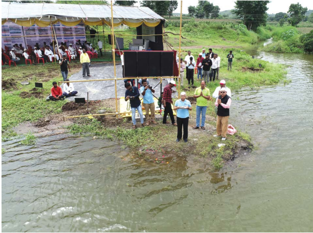
Desilting of Ponds at 20 Sites of 17 villages in Nandgaon Block, Nashik, Maharashtra
