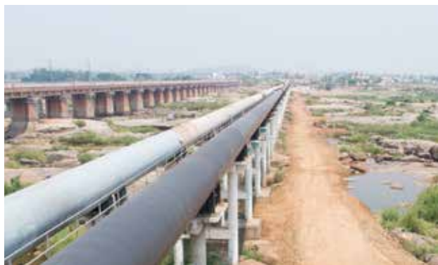
1600 mm dia MS pipeline laying for KPCL Bellary Thermal Power Plant, in Karnataka
