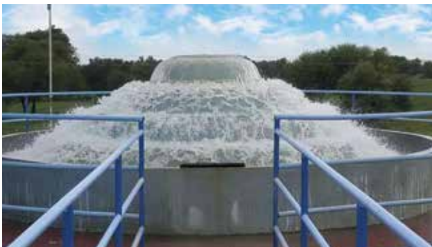
Water Treatment Plant Aeration Process - Aerator for Bankpura Multivillage Rural Water Supply Scheme in Rajgarh Dist., in Madhya Pradesh.
