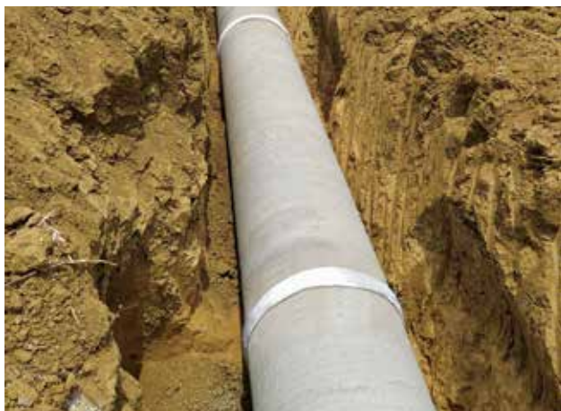
1100 mm dia PCCP pipeline for Asolamendha Project Renovation Division Saoli, Kapsi Branch, in Maharashtra.
