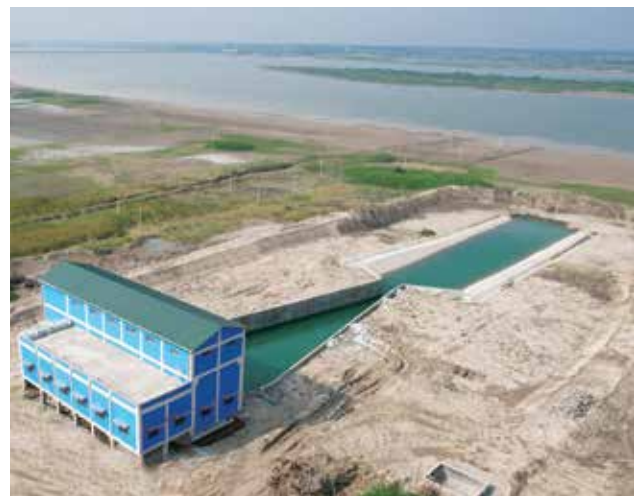
Jack Well Cum Pump House for Minor Irrigation and Ground Water Development Division, Koppal Kushtagi, in Karnataka
