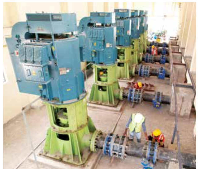
Installation of Pumping Machines at for Minor Irrigation and Ground Water Development Division, Koppal Kushtagi, in Karnataka
