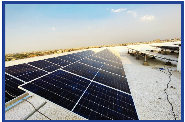
Torrent Power - 341 kW
