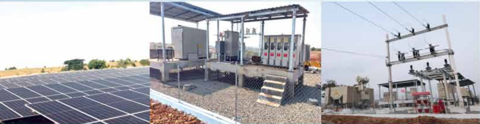
Open Access Captive Generation 6 MWp(DC) Solar Plant Rawankola, Maharashtra
