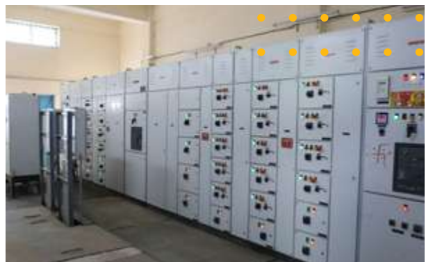
Khan Nagar Pumping Station Panel Room
