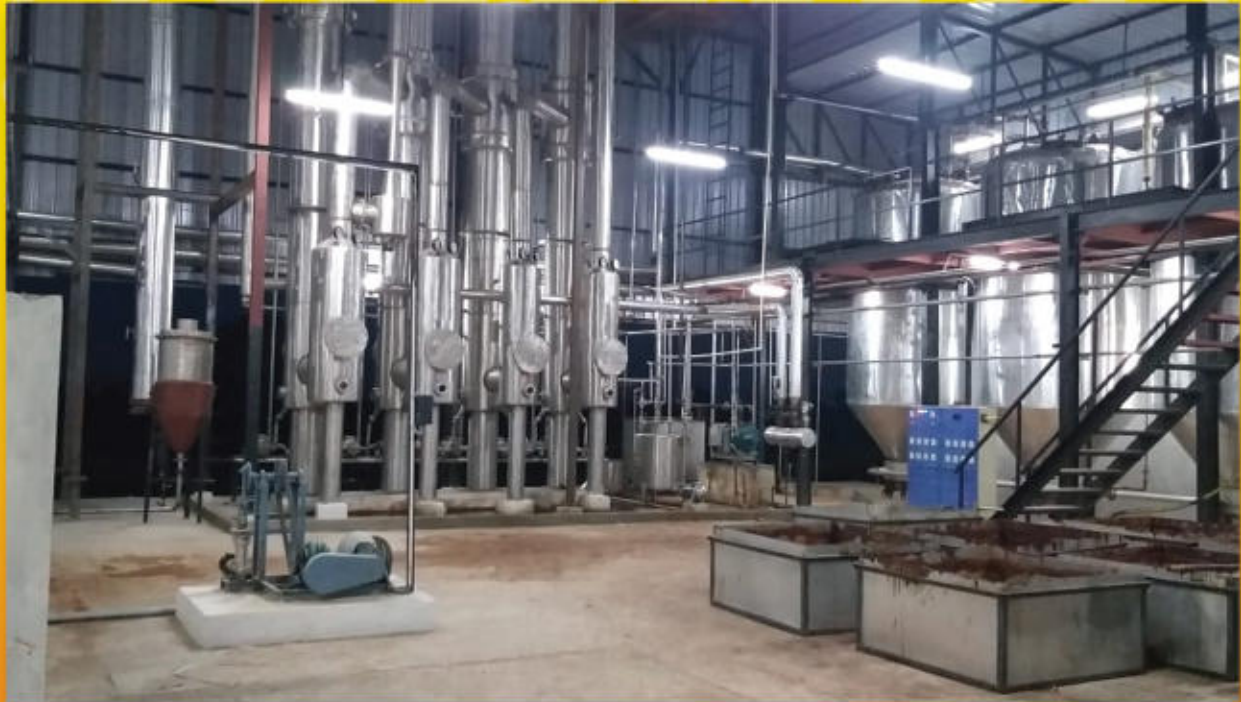
Plant at Jammu
