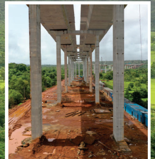
The elevated corridor consists of numerous piers that reach height of up to 40 meters.
