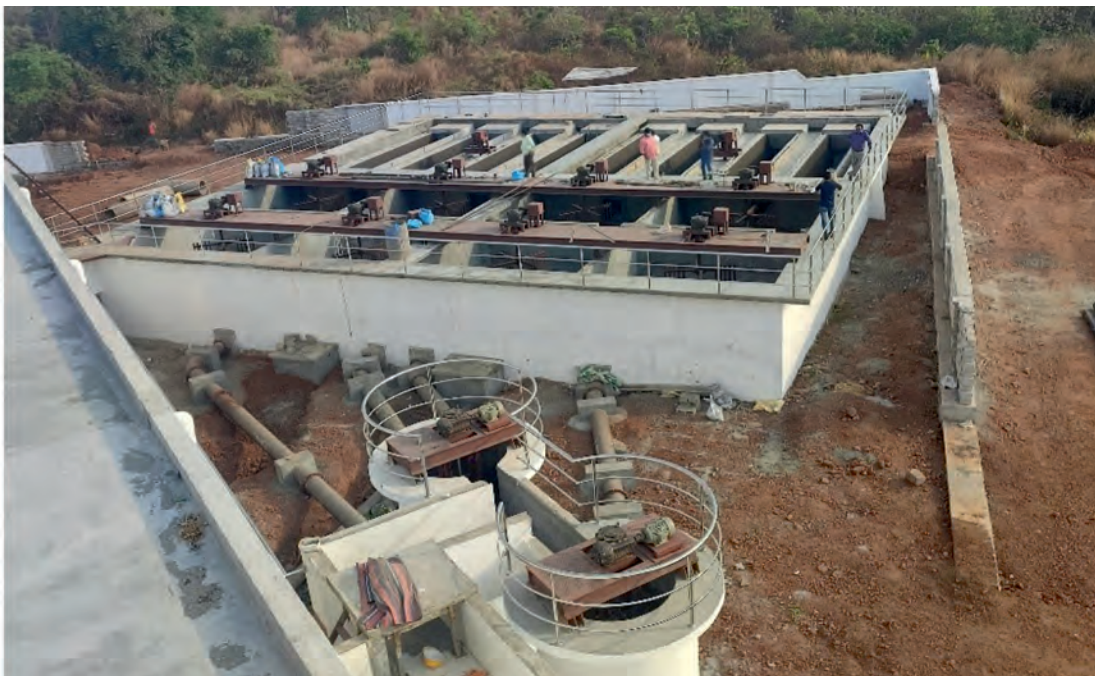
Water Treatment Plant at Kondotty Municipality, Kerala
