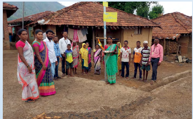
Inauguration pooja by villagers and FIL members for solar lights – Palghar, Maharashtra
