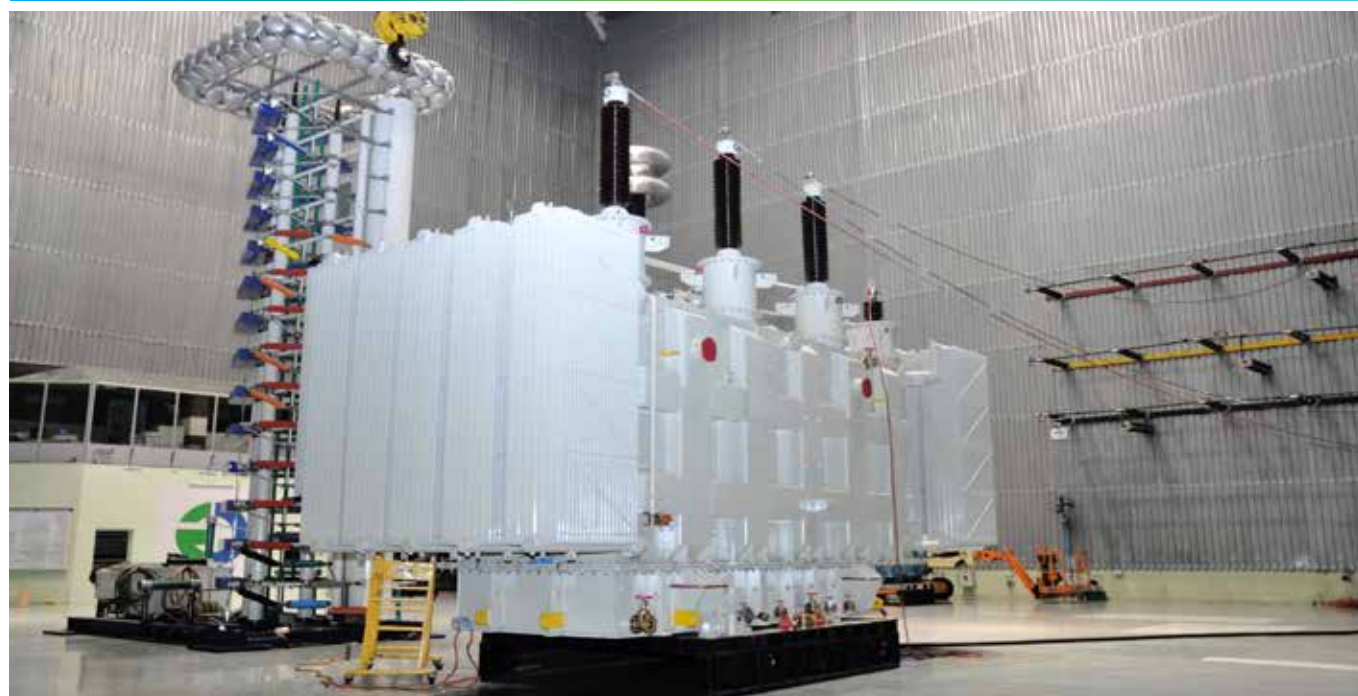
160MVA, 220kV TRANSFORMER
