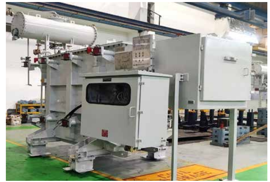
T2 - Transformer 8MVA 13.8kV
