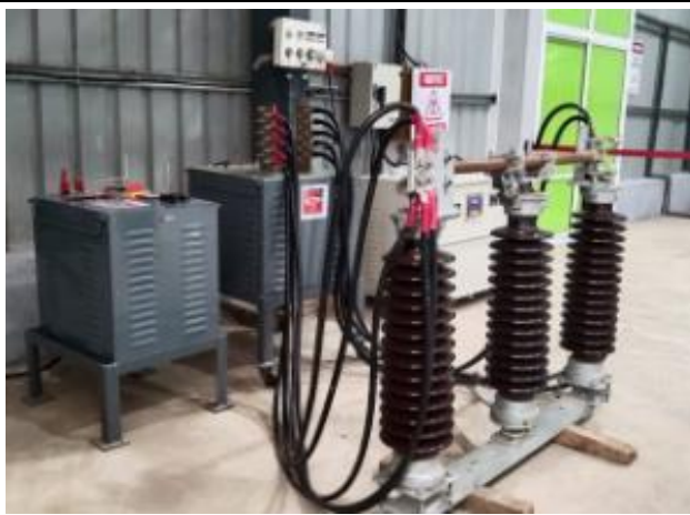
HV DISCONNECTOR STRUCTURE
