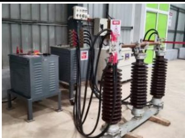
HV DISCONNECTOR STRUCTURE
