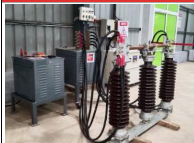
HV DISCONNECTOR STRUCTURE
