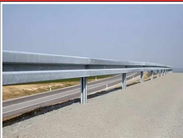
METAL BEAM CRASH BARRIER
