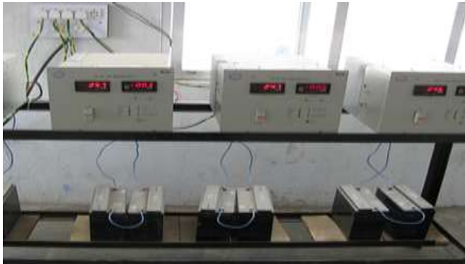
Battery and Battery Chargers
