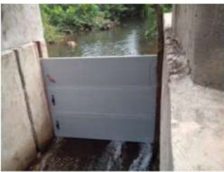
FRP Dam Doors
