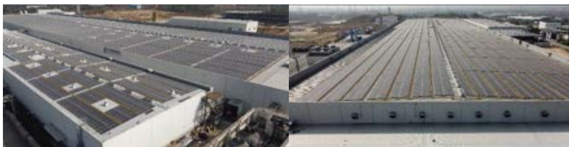
6.61 MW solar rooftop plant
