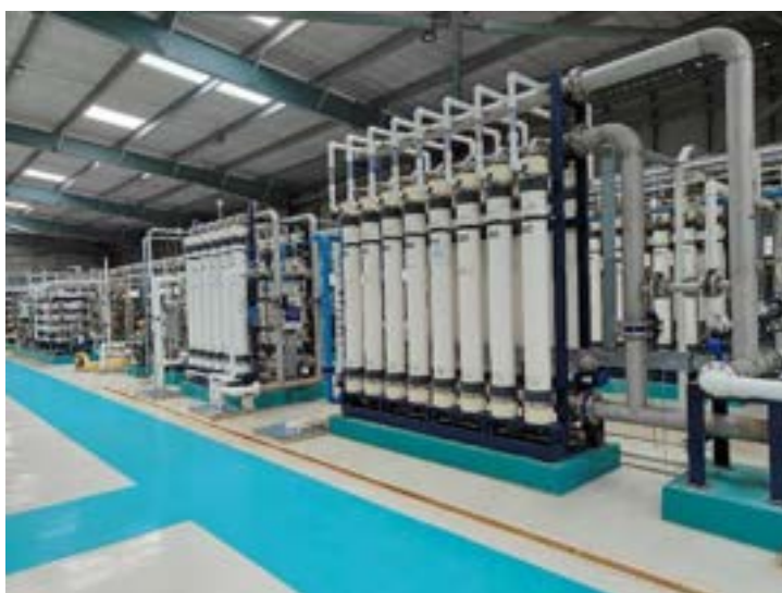
Ultra-pure water generation plant at Unit II
