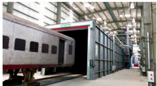
Stainless Steel Cut Wire Blast Plant at Modern Coach Factory, Raebareli
