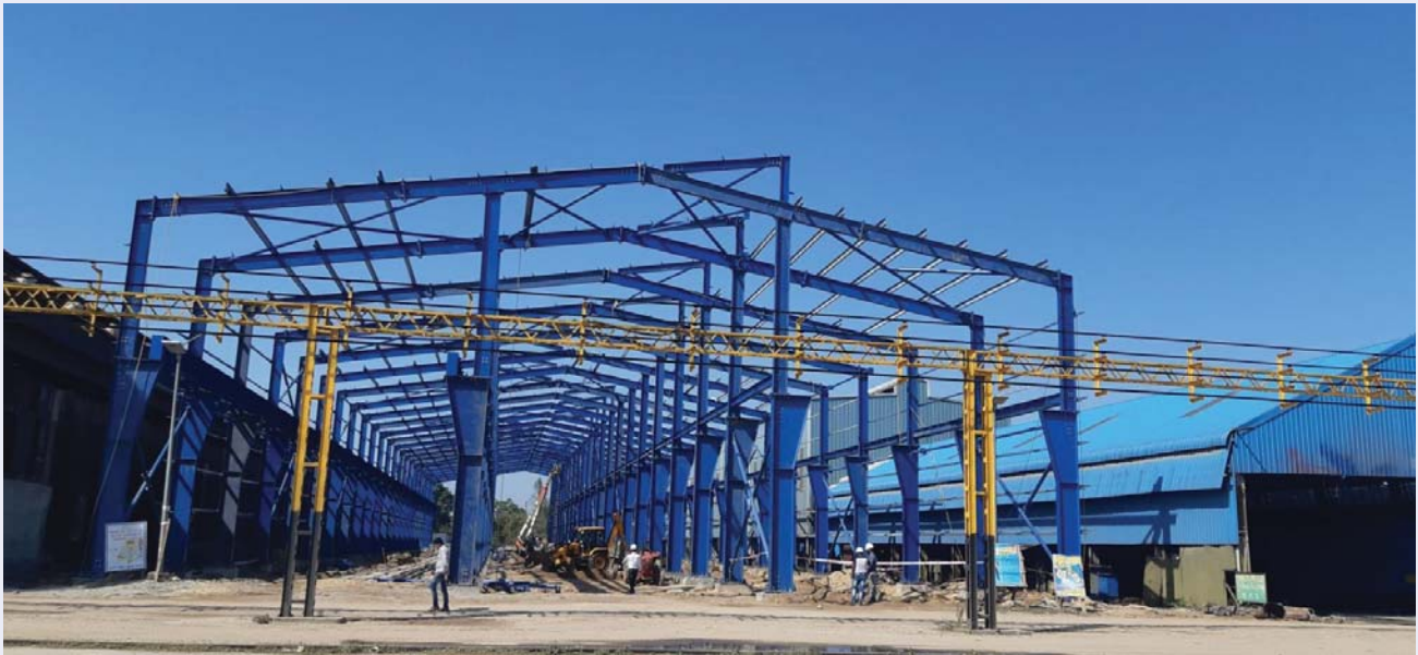
Setting up of workshop for refurbishing LHB coaches at New Bongaigaon, Assam
