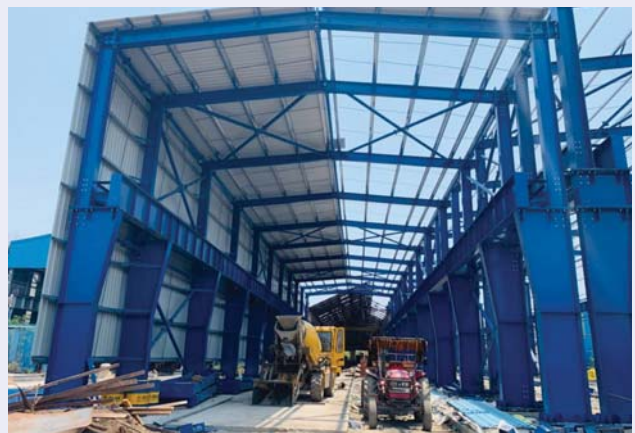
Facilities for augmenting periodical overhauling capacity from 20 to 120 BG wagons per month at Kurduwadi Workshop, Maharashtra
