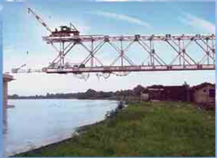
Bhairab Bridge, Bangladesh Assembly of a 102.4 M length span Girder (one of the 9th spans) at Panihati Works. The total length of the Bridge is 1.02 km.
