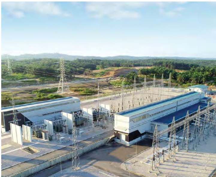
275/132/33kV Gas Insulated Substation, Samalaju, Malaysia
