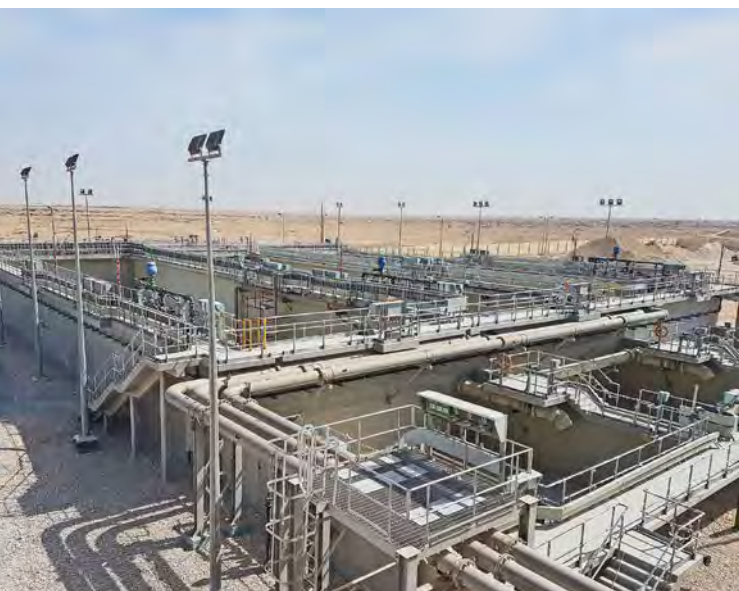
Al Shammal Water Treatment Plant at Qatar
