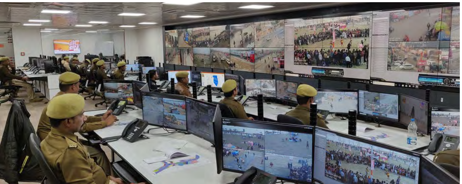
L&T's Integrated Command & Control Centre managed traffic, people movement and surveillance of over 20 crore pilgrims at the Kumbha Mela
