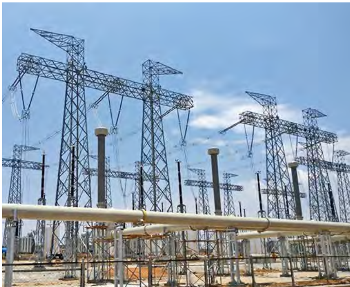
765 kV Gas Insulated Substation, Hyderabad
