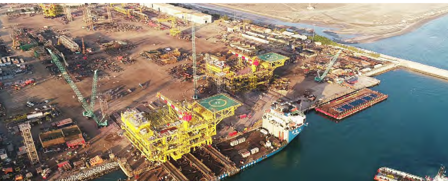
Load-out of two mega Tie-in Platforms (7000 MT each) for Hasbah Field, Saudi Aramco from L&T Hydrocarbon Engineering's Oman facility
