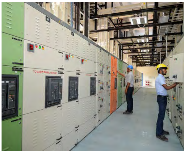
Switchboard installation at a national infrastructure site
