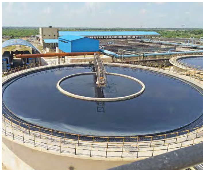
Common Effluent Treatment Plant, Narol
