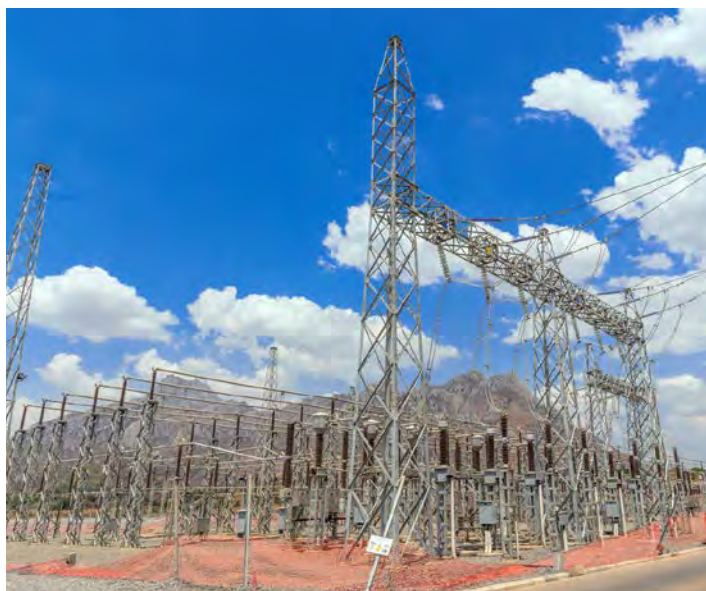
400/132kV Substation, Nkhoma, Malawi
