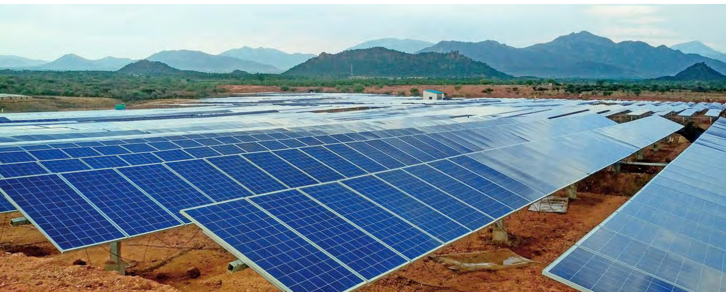
55 MWp Solar Tracker Plant at Theni, Tamil Nadu
