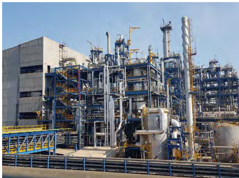
40,000 MTPA Melamine Plant for Gujarat State Fertilizers & Chemicals, Vadodara, India
