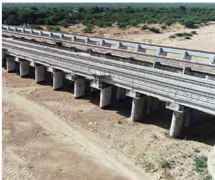
A rail bridge on the Western Dedicated Freight Corridor section being built by L&T
