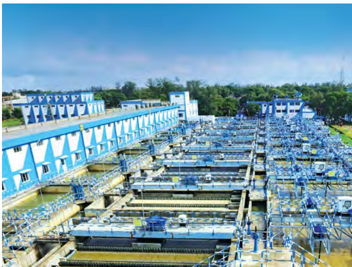
227 MLD Water Treatment Plant, Kolkata, West Bengal
