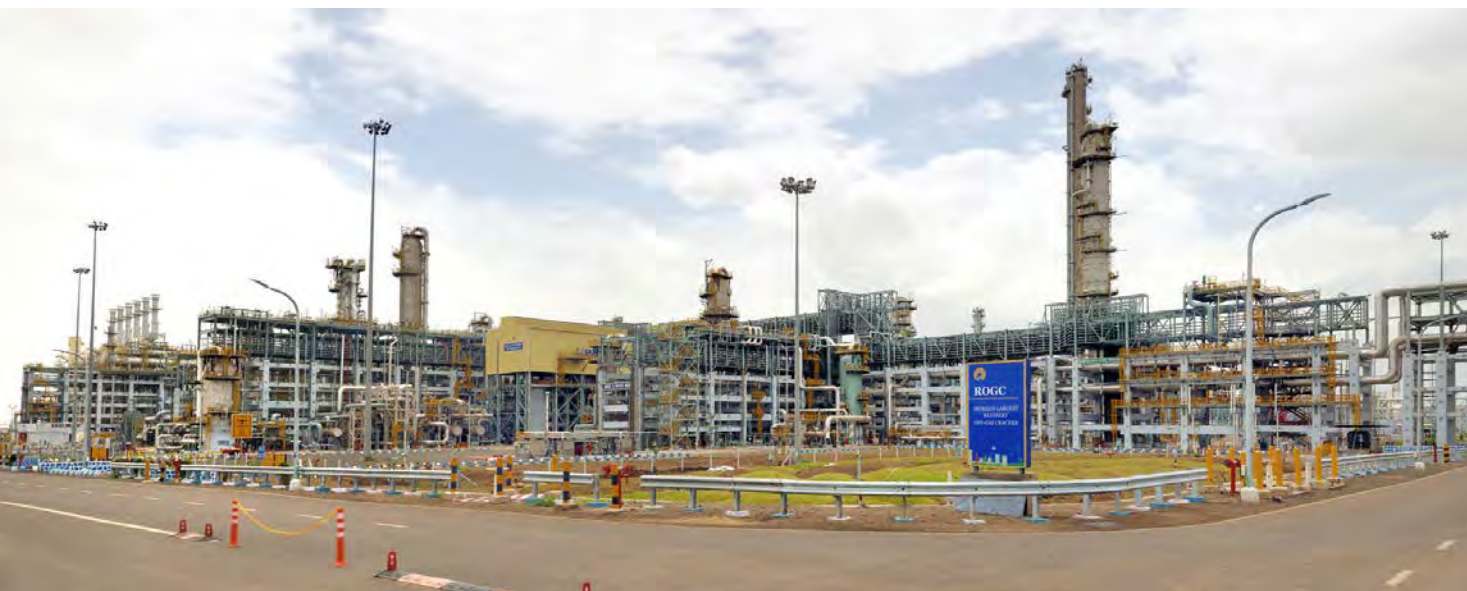
Construction of the world's largest ethylene cracker (1.4 MMTPA) for Reliance Industries, Jamnagar, India
