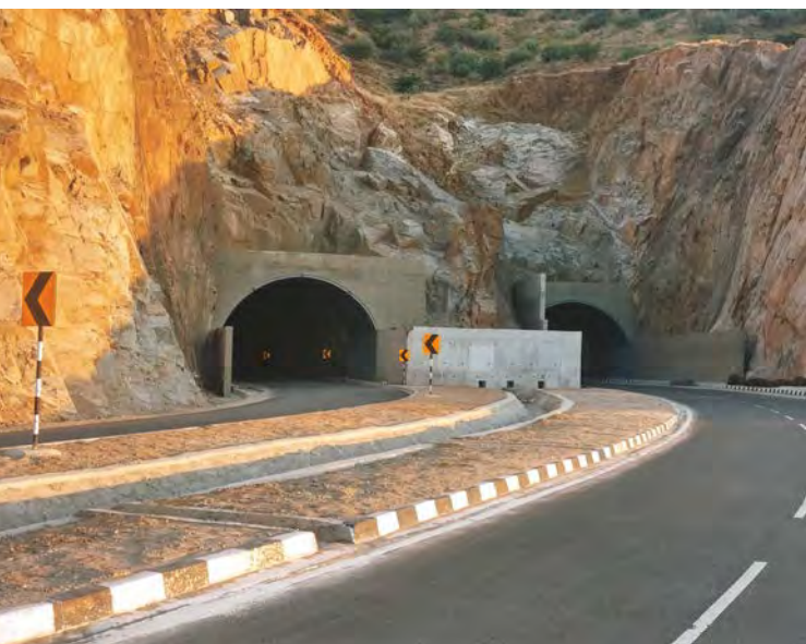
The 221.4 km Beawar – Pali – Pindwara road in Rajasthan is the longest four lane road project developed under the (PPP) model in the National Highways sector.
