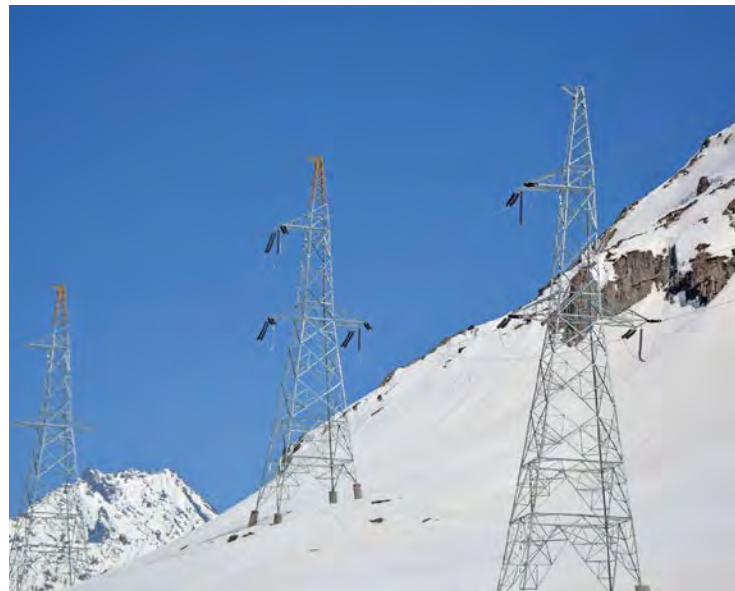
220 kV Alusteng-Drass Transmission Line, Jammu
