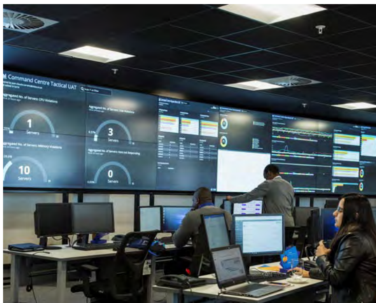
LTI's state-of-the-art Delivery Centre in Johannesburg, South Africa
