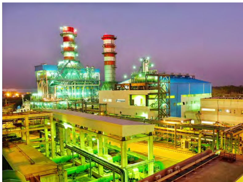
225 MW Sikalbah Combined Cycle Power Plant, Bangladesh
