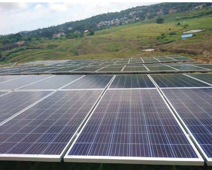
Large scale solar cum storage project in Andaman
