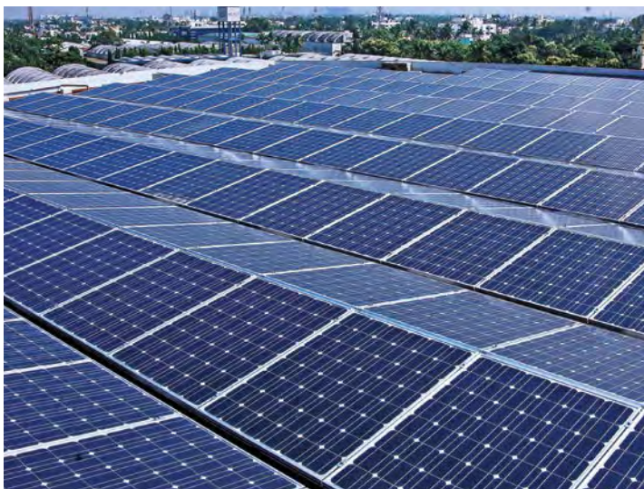
Alternative energy sources at L&T campuses help lower the Company's carbon footprint
