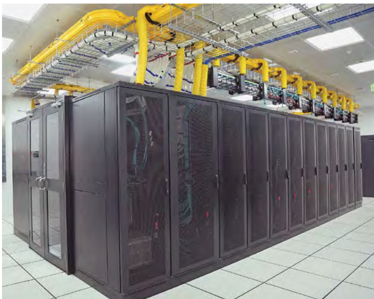
Data Center, Hyderabad
