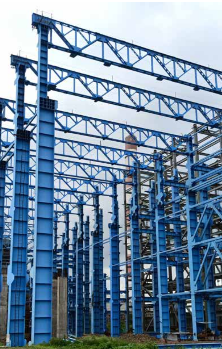
1X660 MW Bhusawal TPS, Maharashtra
