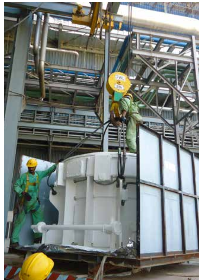
2X 660 MW Singareni Thermal Power Plant at Telangana
