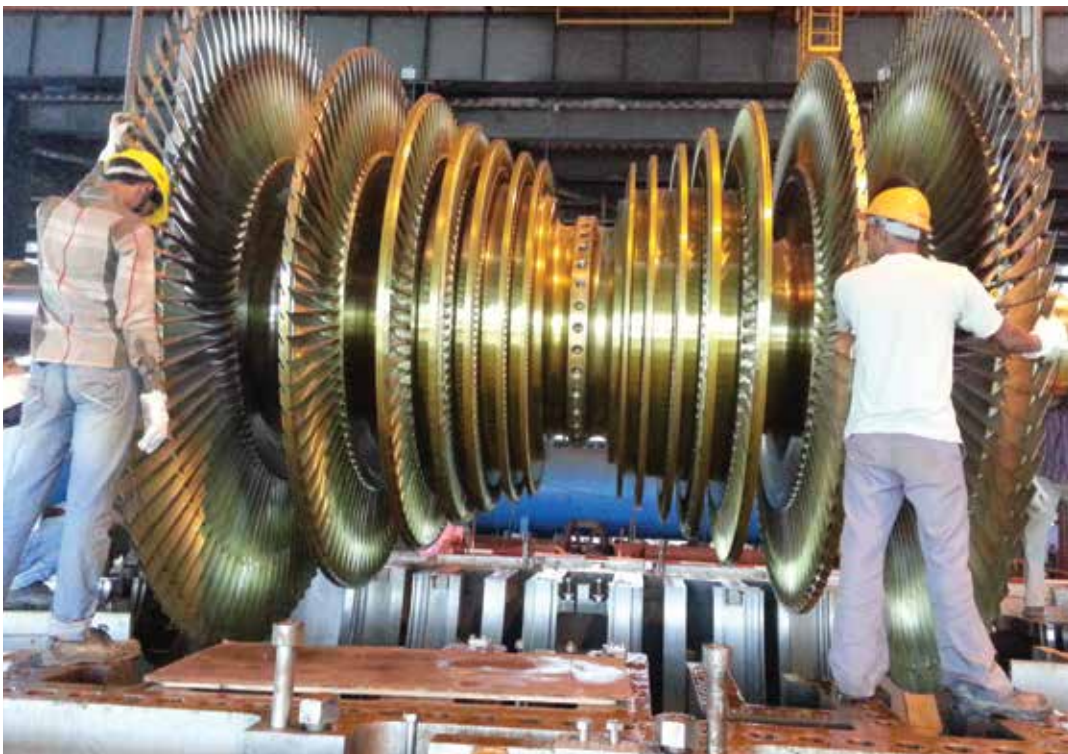
LPT 106 MW STG at NTPC Auriya, UP
