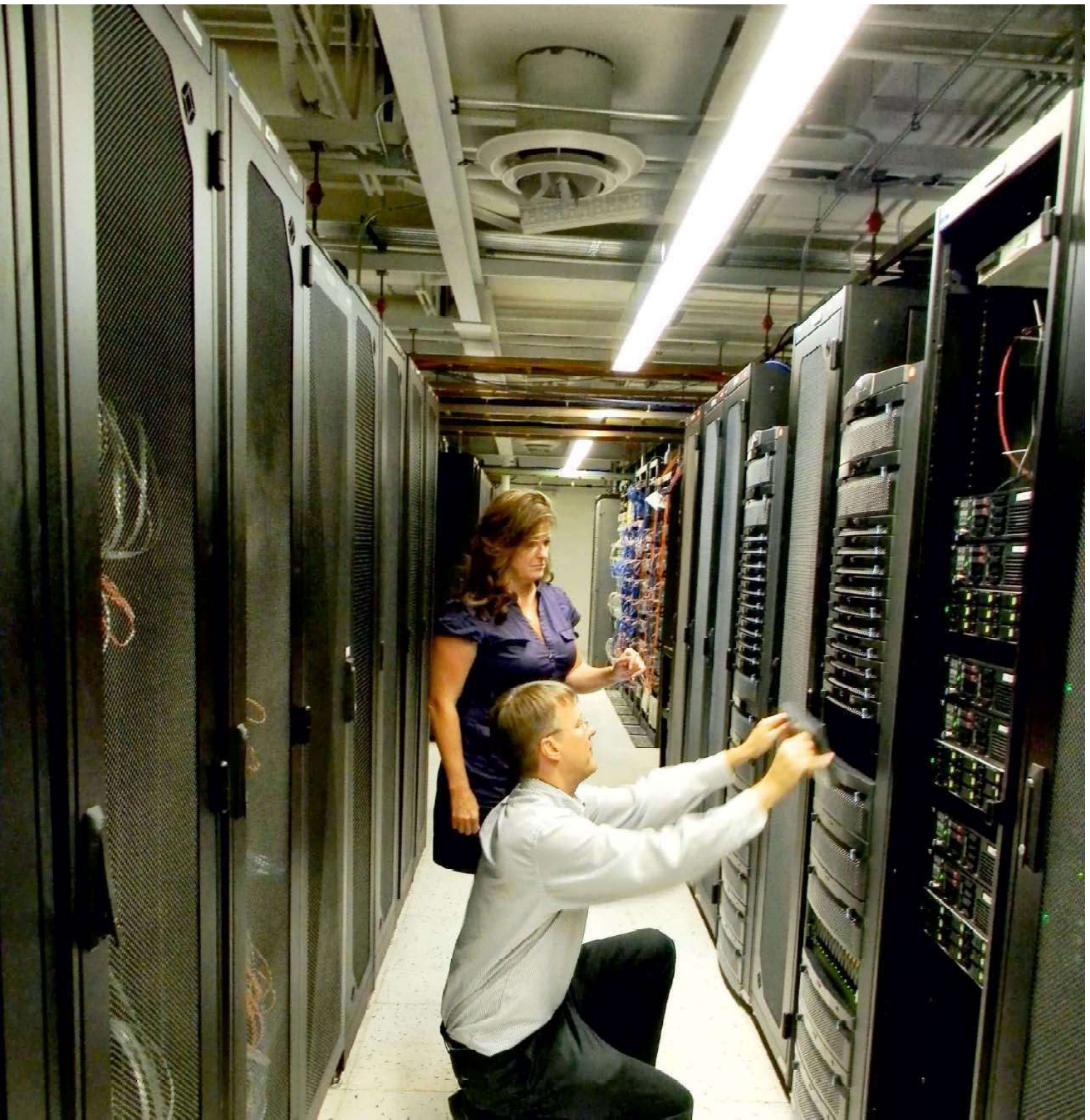
Mobility & Messaging Lab | Rockville, MD, USA | 5000 sq. ft. | 22 Racks, >50 Servers
