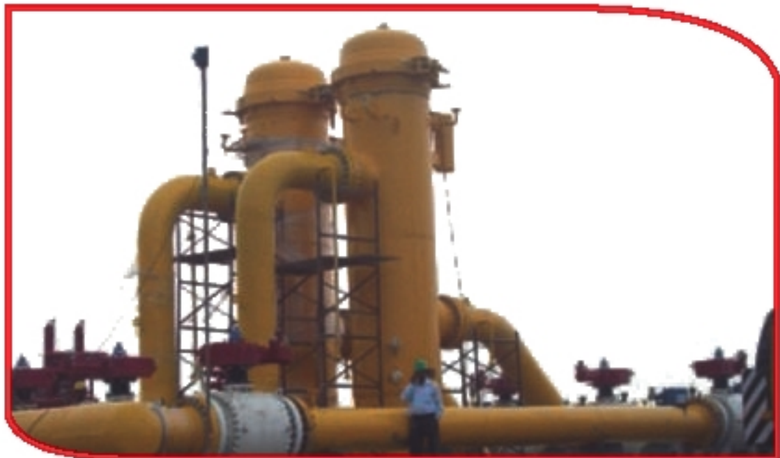
Ad's largest metering skid erected by Moyas Infra Limited at Jamnagar in record time
