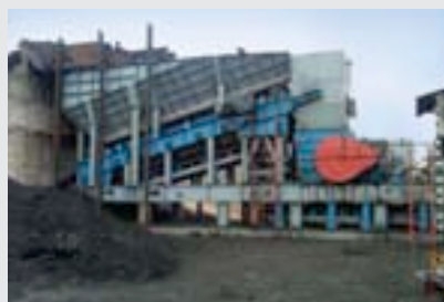
Skid mounted Coal crushing plant
