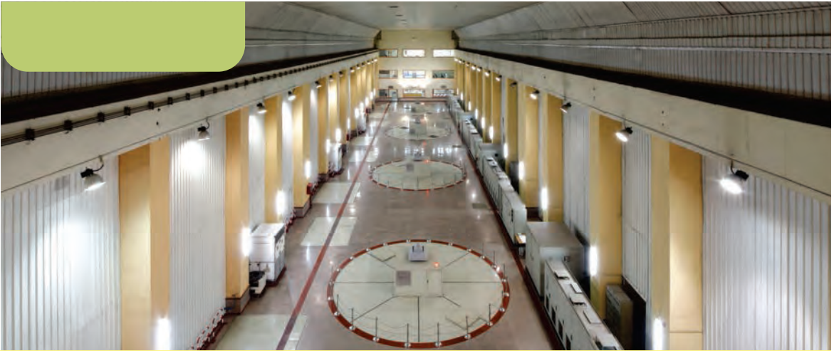
400 MW Vishnuprayag Powerhouse, Uttarakhand
