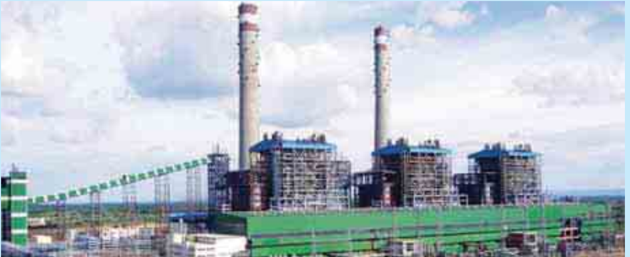
1980 MW Bara Thermal Power Project, Allahabad, Uttar Pradesh (To be fully commissioned within FY 2016-17)
