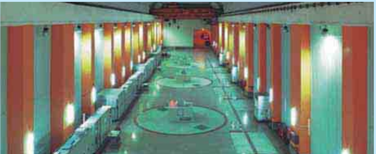
400 MW Vishnuprayag Powerhouse, Uttarakhand
