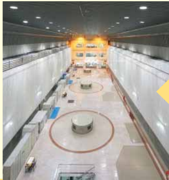
Machine Hall at 300 MW Baspa-II Hydro Electric Power Plant, Himachal Pradesh
