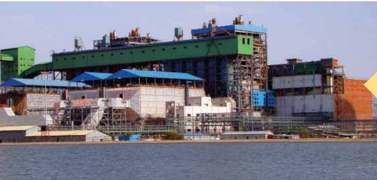
View of ESP, bunker and boiler with water reservoir in foreground at Bina TPP, Madhya Pradesh
