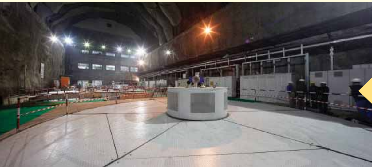
Machine Hall at 1000 MW Karcham- Wangtoo Hydro Electric Power Plant, Himachal Pradesh
