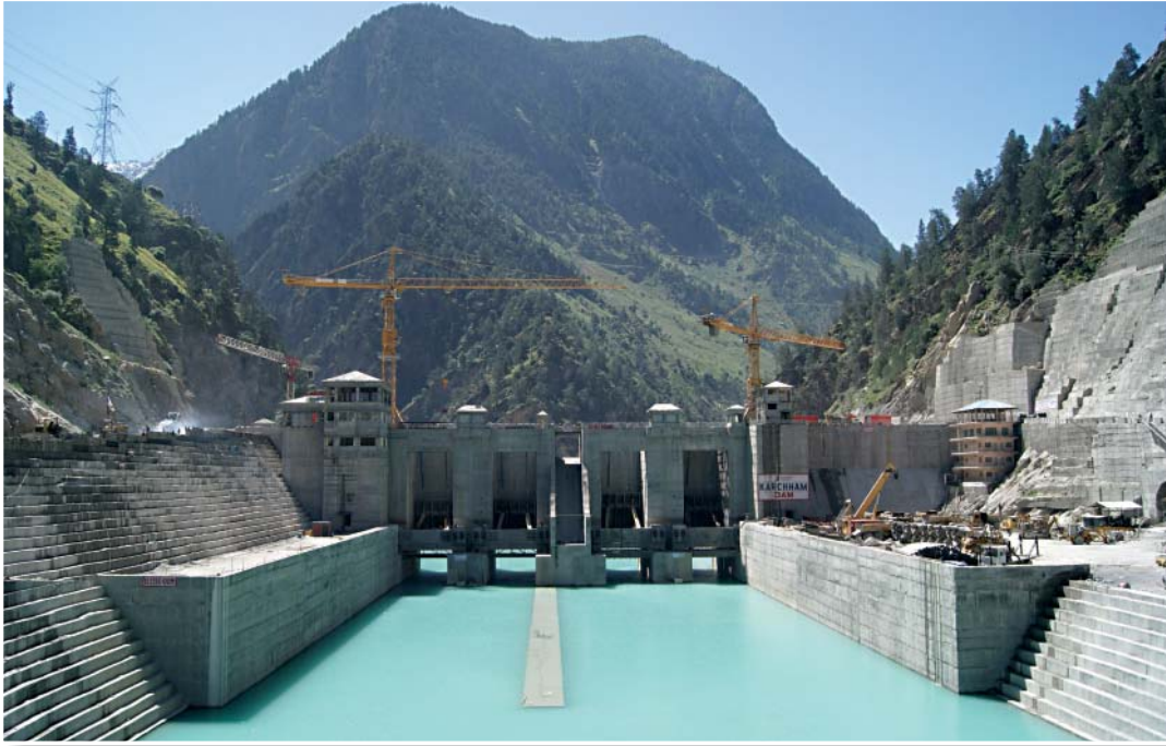
1000 MW Karcham Wangtoo Hydro Power Project, Himachal Pradesh
