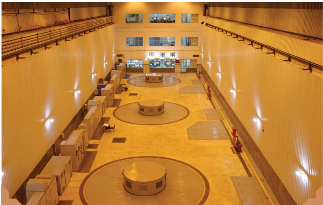
Machine Hall at 300 MW Baspa-II Hydro Power Station, Himachal Pradesh
