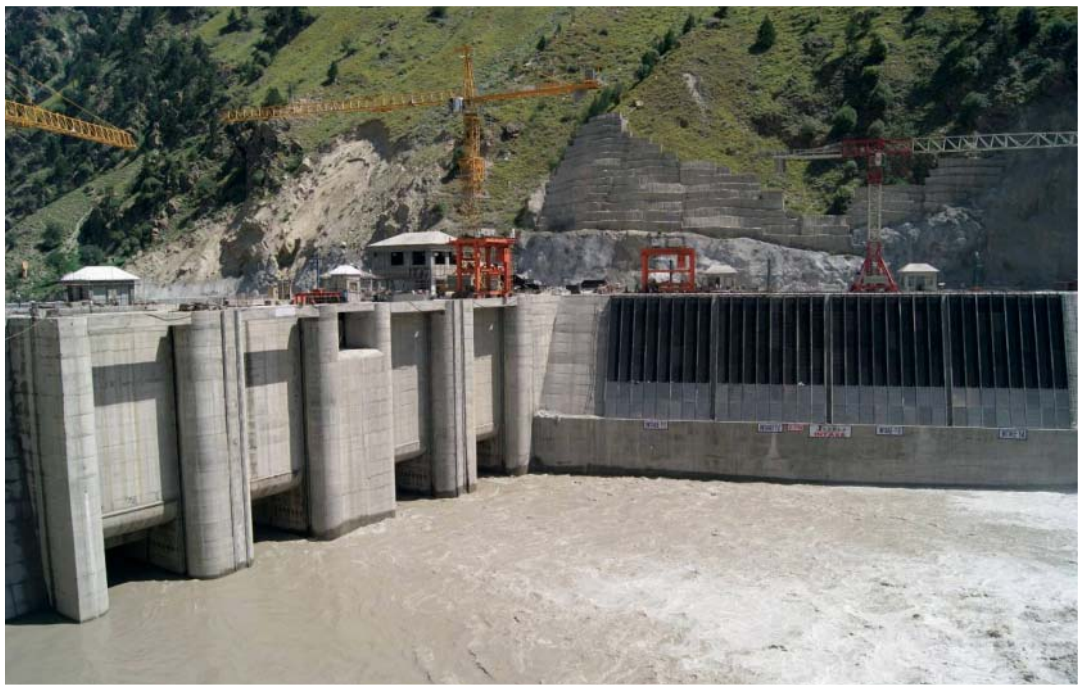
View of inlet at 1000 MW Karcham Wangtoo H.E.P., Himachal Pradesh
