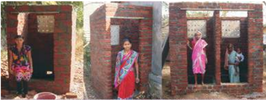
Some of the ongoing toilet construction works from Shahapur Taluk, Thane Dist.
