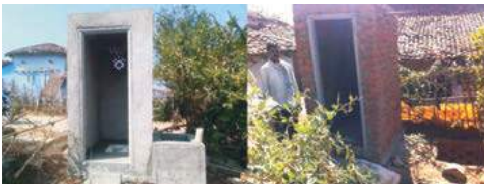
Construction of toilets in Ramtek block of Nagpur District, Maharashtra in progress
