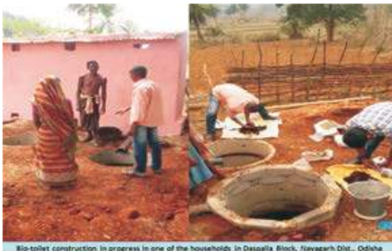
Bio-toilet construction in progress in one of the households in Daspalla Block, Nayagarh Dist., Odisha
