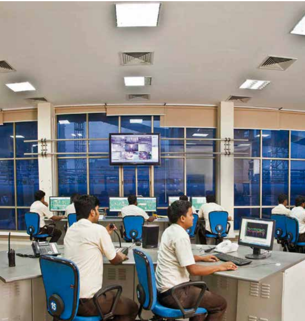
Central control room, PM6 - Unit JKPM
