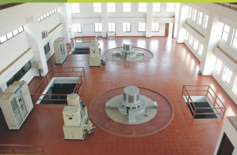
The Prestigious Hydro Power Project At Radhanagaeri (Internal View of Turbines)
