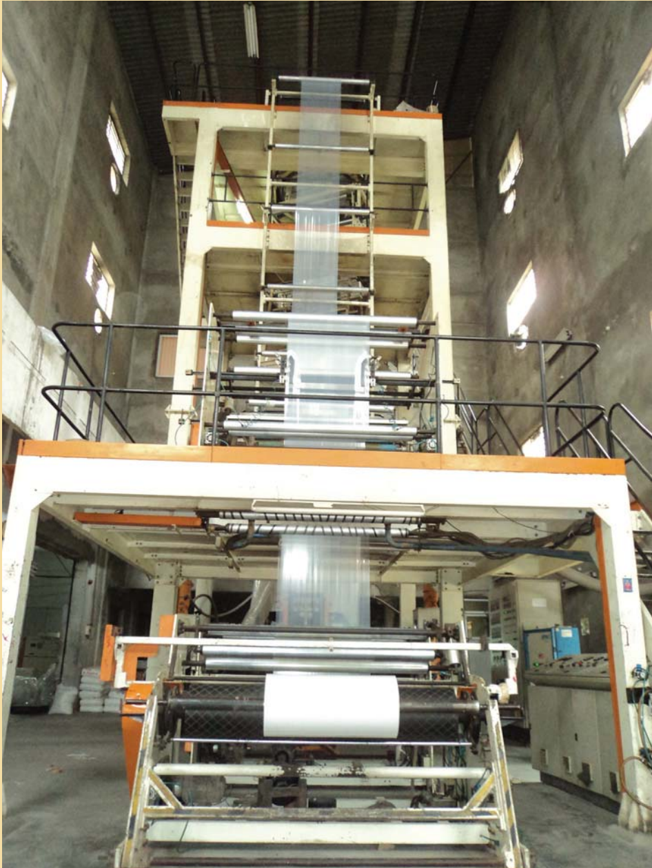
3 Layer Blown Film Plant
