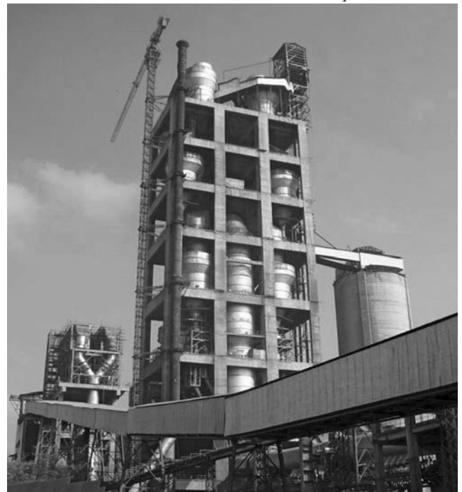
Preheater Structure at Chandrapur, Maharashtra
