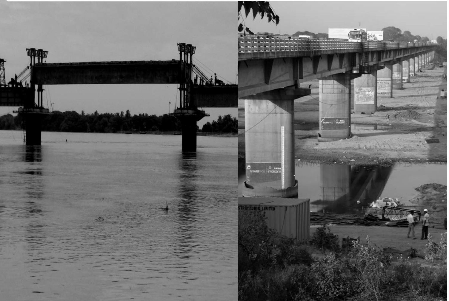
Precast Prestressed Girder of 43.5m span being erected for Railway Bridge on Luna River in Orissa for M/S RVNL
