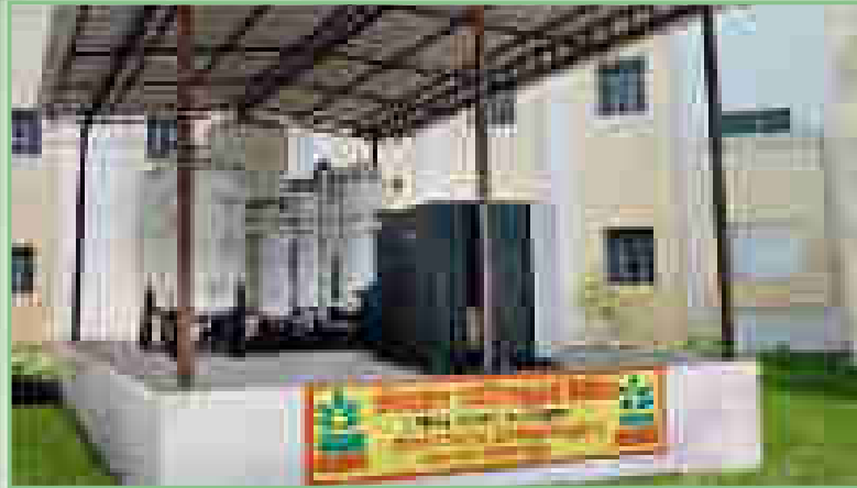
The company installed & commissioned 04 nos. Medical Oxygen Generator Plants at Bhopal, Lucknow, Gorakhpur & Indore to strengthen the Covid Care facilities
