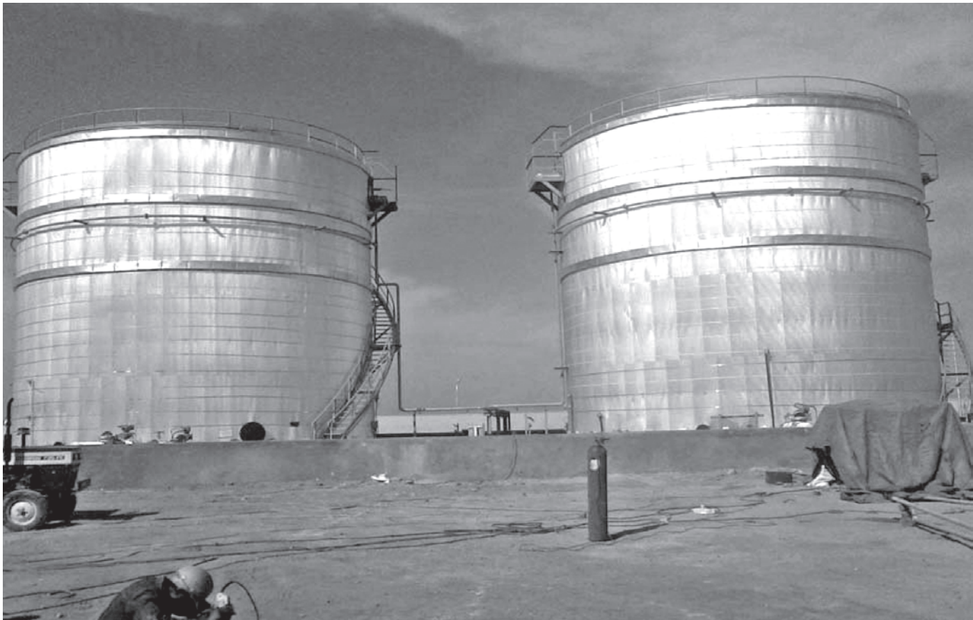
▲ Crude Oil Tanks, Radhanpur
