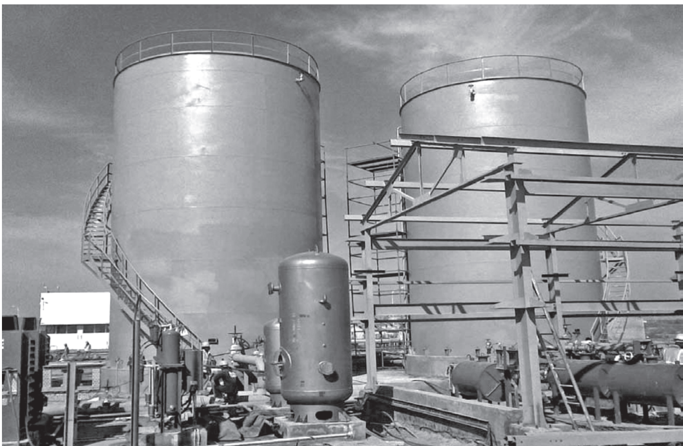
Fire Water Tanks, Radhanpur ▼
