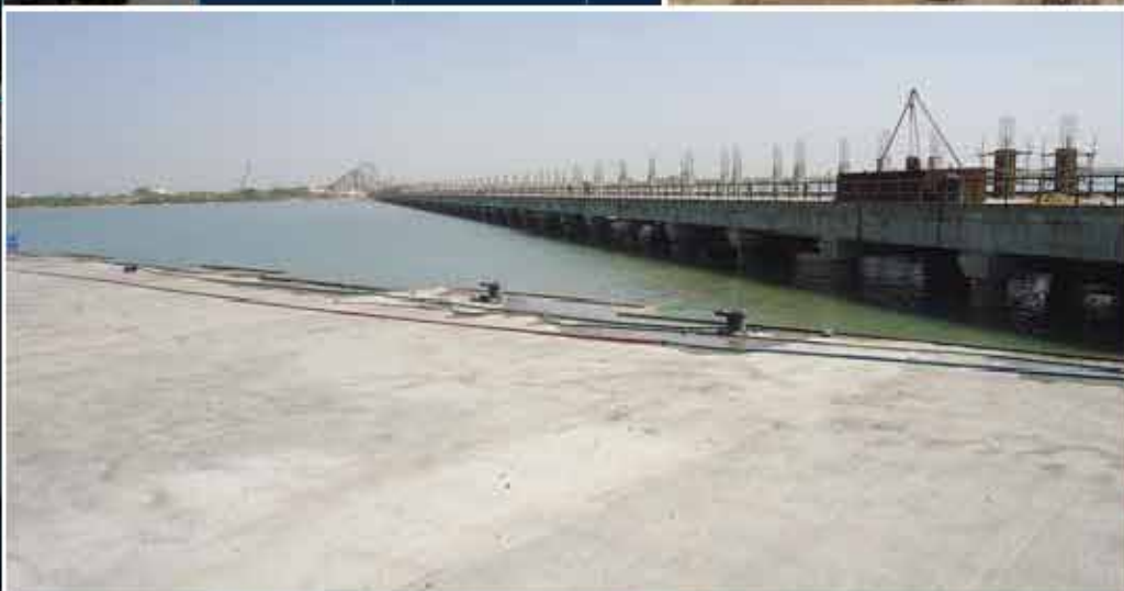
Jetty for Jaypee Cement at Gujarat
