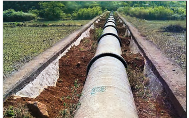
1100 mm dia PSC Pipe line for Vadiwale Left Bank Canal pipe line project Near Pune, Maharashtra
