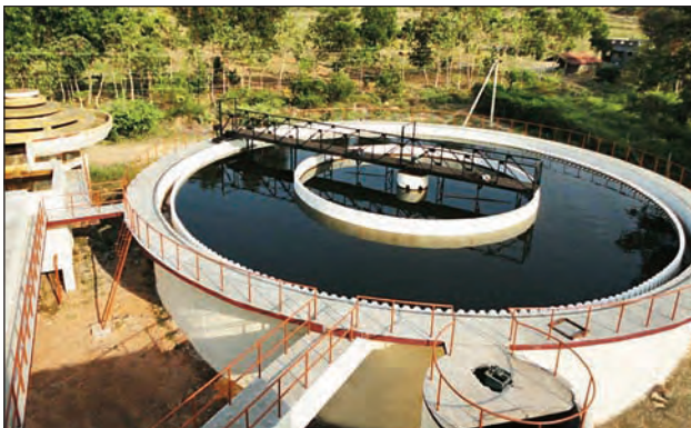
Construction of Aerator & Clariflocculator for 11.75 MLD water treatment plant under the work of CWSS to Madathukulam & other 112 Rural Habitation of TWAD Board, Coimbatore
