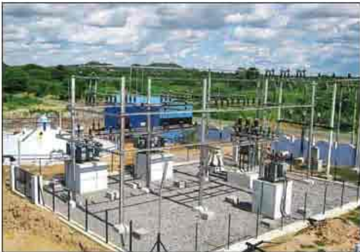
33 KV Sub Station
