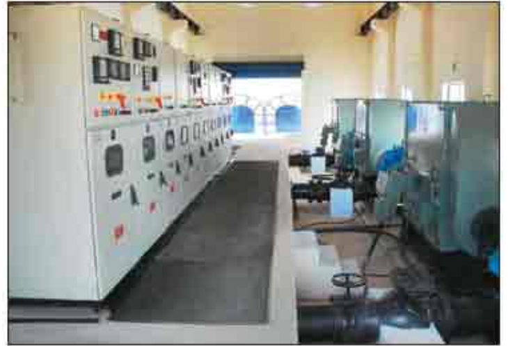
Pumps and Motor
