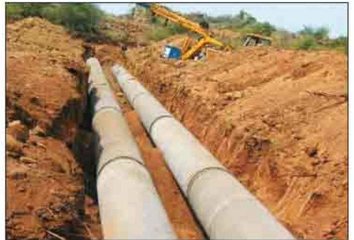
900 mm Dia BWSC & M S Pipe Line (30 KM)
