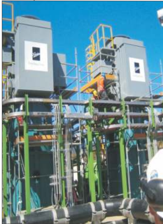
Successful commissioning of 2 Sets of CW pumps for 370 MW Central Thermolectric Santa Maria project at Coronel in Chile of Colbun SA – bowl pull out design pumps for sea water application.
