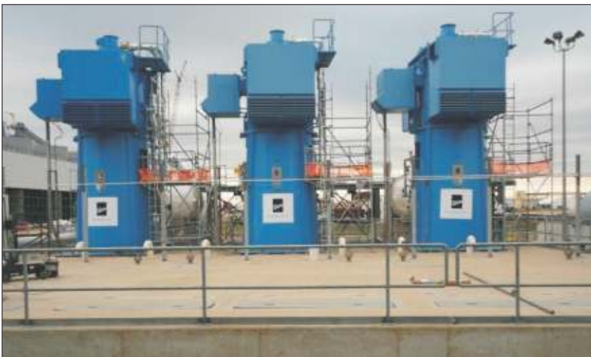
Successful commissioning of 3 Sets of CW pumps for the 2x800 MW Prairie State Energy Campus, Illinois, USA.
