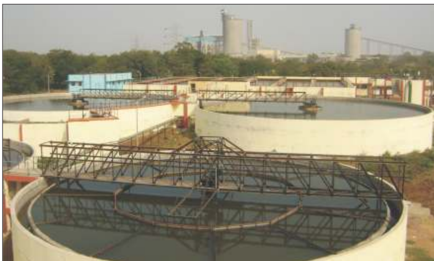
125 Million Litres Daily (MLD) water treatment plant for Coimbatore Municipal Corporation
