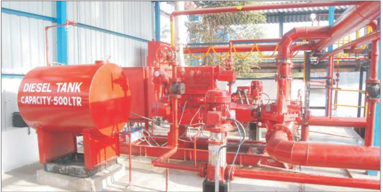
FM / UL fire hydrant system erected and commissioned at Jindal Steel and Power Limited, Raigarh (Chattisgarh)
