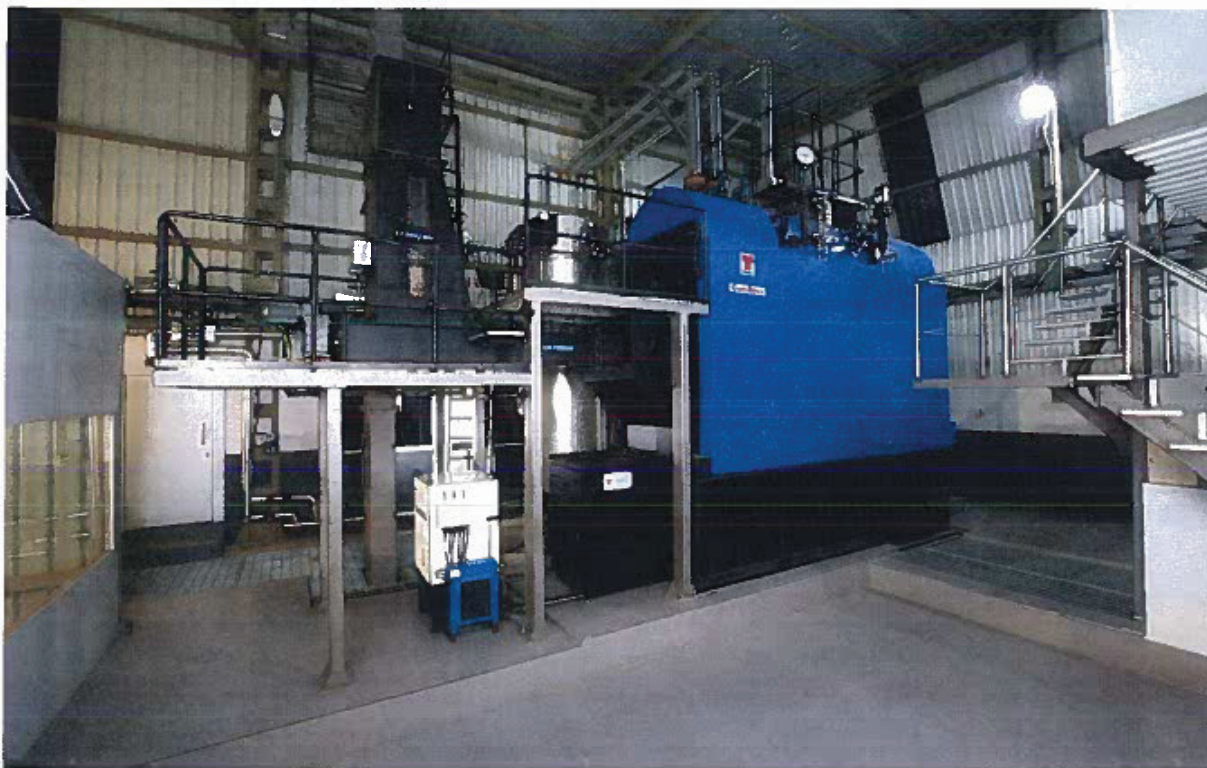
Biomass fired boiler Combloc CB-20 (2tph) installed at Thermax factory, Pune
