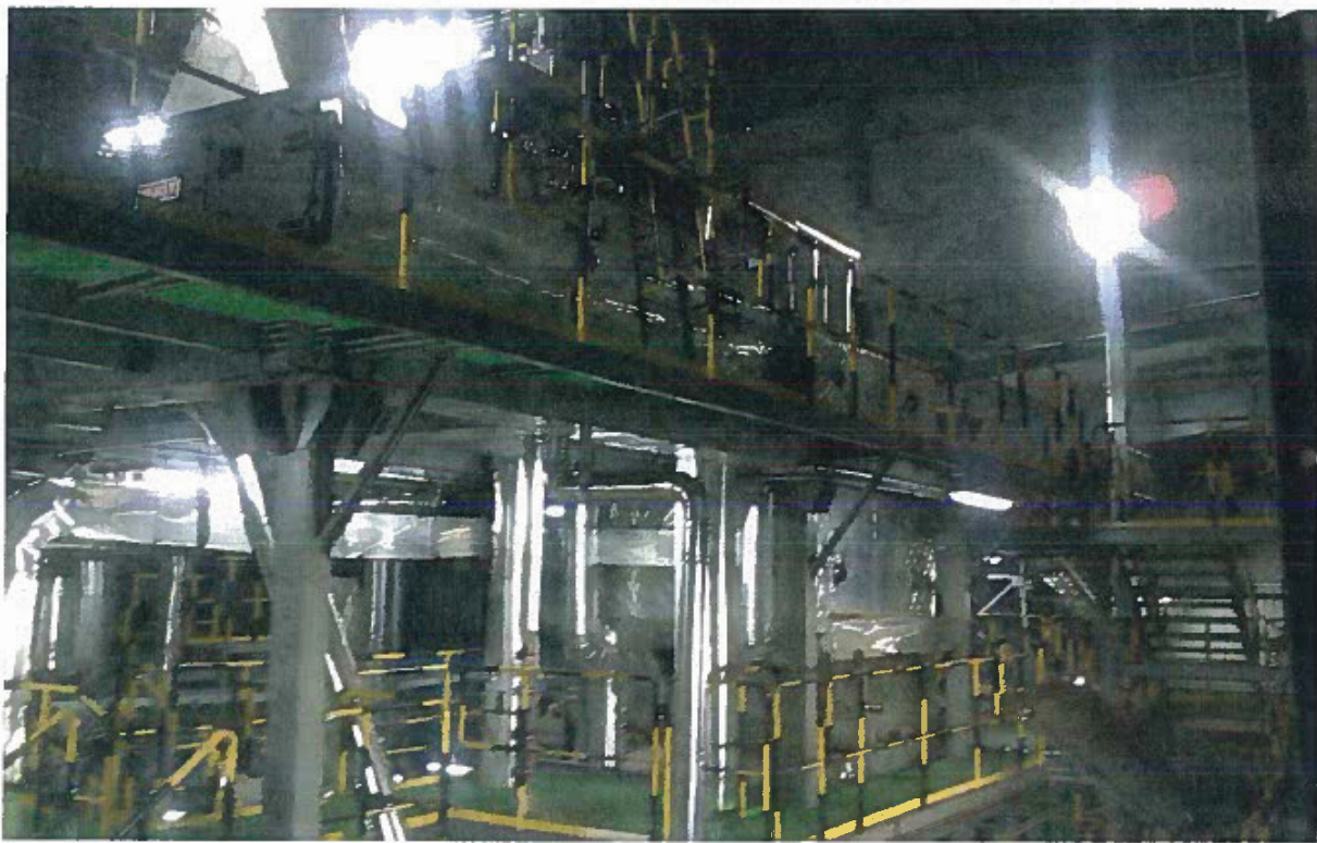
Installation at Hosur, Biomass fired Boiler - CPRG-60 (6tph)
