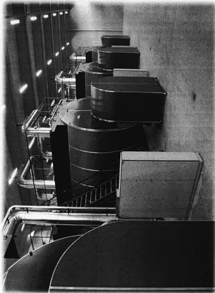
Gas fired boilers for District Heating
