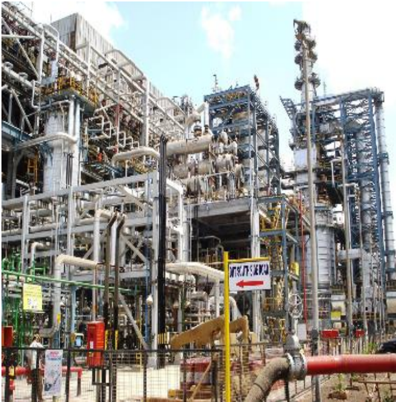
Mumbai Refinery - 1.76 MMTPA
