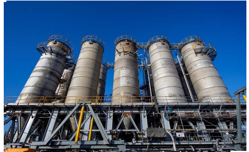
Rajasthan: Polymer Storage Silos
