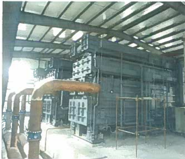
3 x 30 MW Absorption Heat Pumps for District Heating application at Harbin, China
