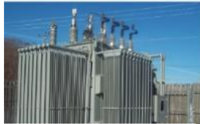
Transformer & Sp Oil
